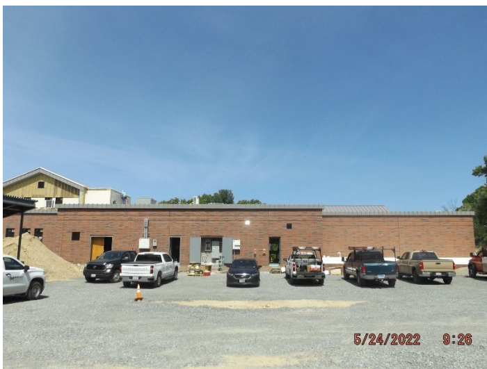
Photo depicts the progress of the exterior at the rear of the fire department side.
