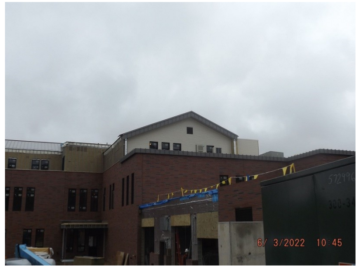
Photo depicts the progress of the sally port overhead door framing and installation of hardi plank siding.
