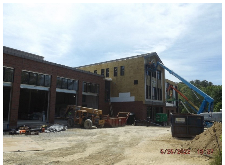
Photo depicts the progress plywood sheathing and avb for the metal siding.
