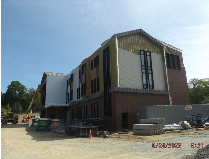
Photo depicts the progress of installation of hardi plank siding, avb over the plywood sheathing for the metal siding.
