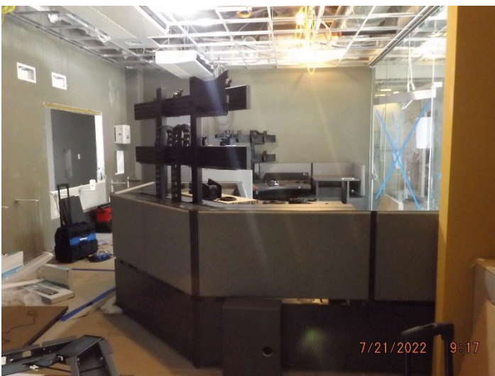
Photo depicts the progress of dispatch consoles.
