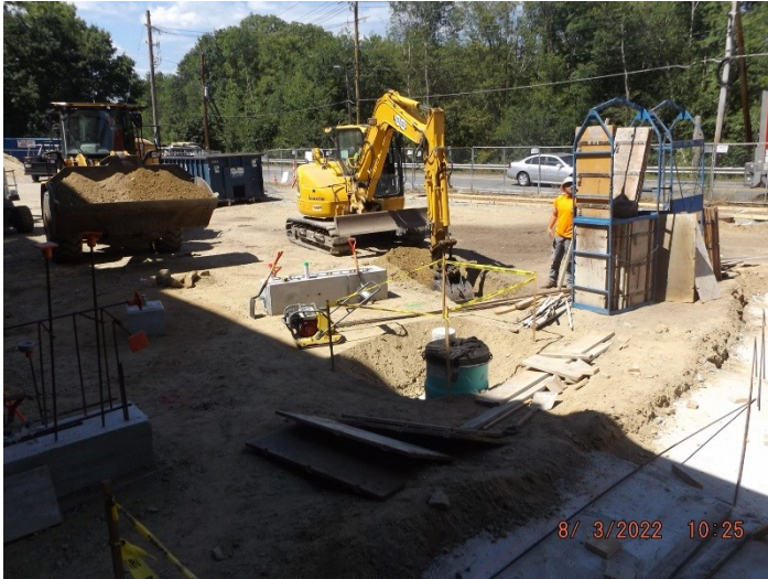
Photo depicts the progress of entry ramp and stairs along with site lighting.
