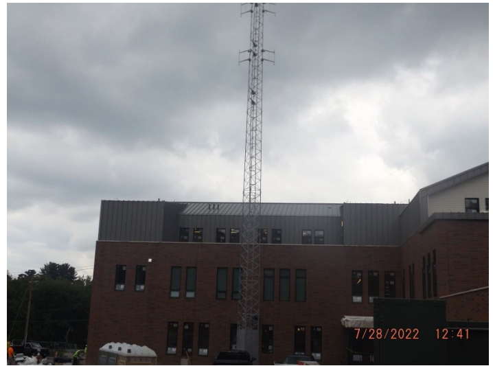
Photo depicts the progress the rear of the admin side of the building.
