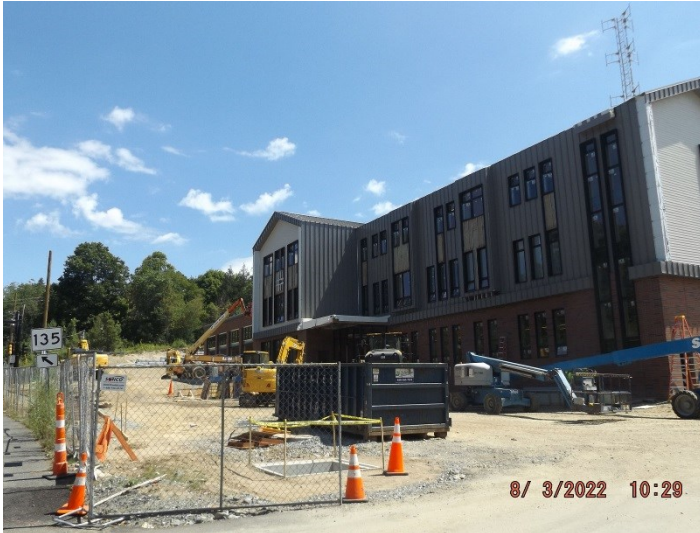
Photo depicts the progress of installation of the standing seam metal siding and progress of the site work out front.
