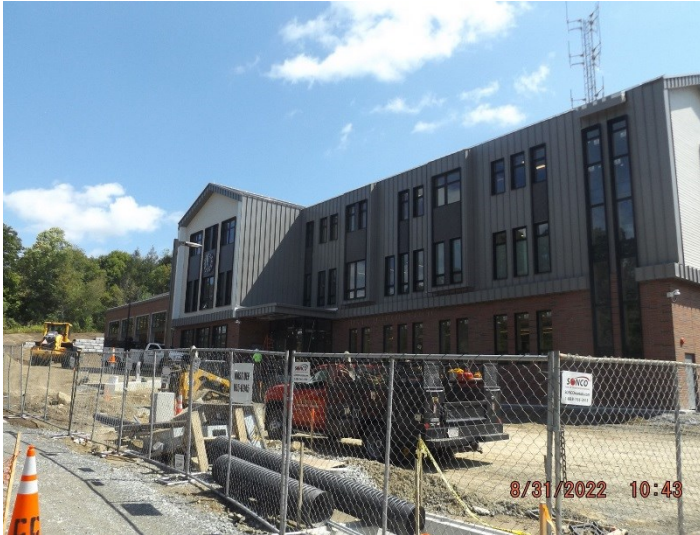
Photo depicts the progress of the front of the site and completed exterior.
