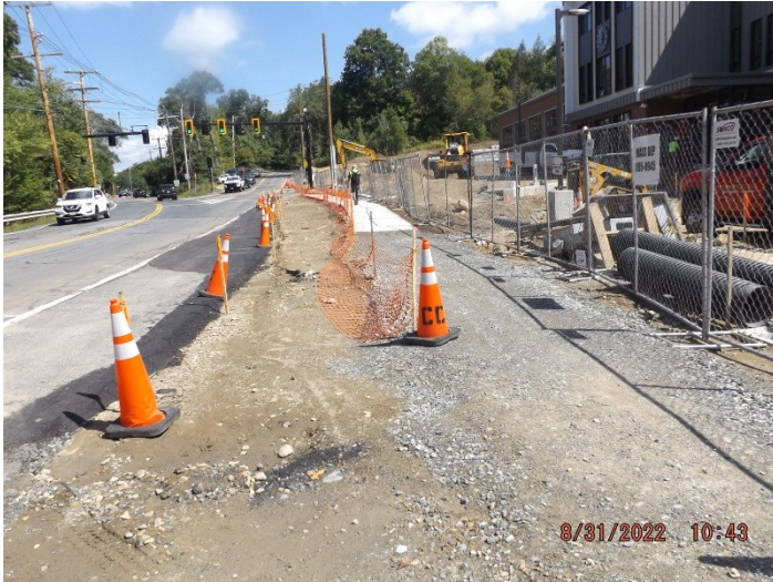
Photo depicts the progress of the widening of the road and new sidewalk.
