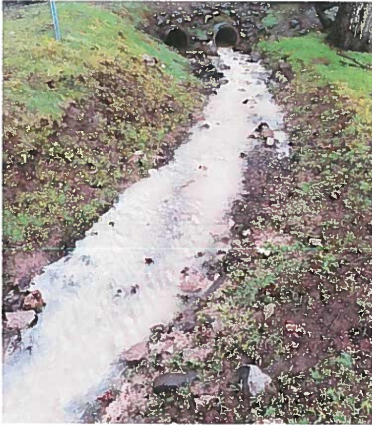
7/2/2021: Picture taken by Jeff Fournier, Plant Operator (water treatment plant). These culverts are under Howe Street.
