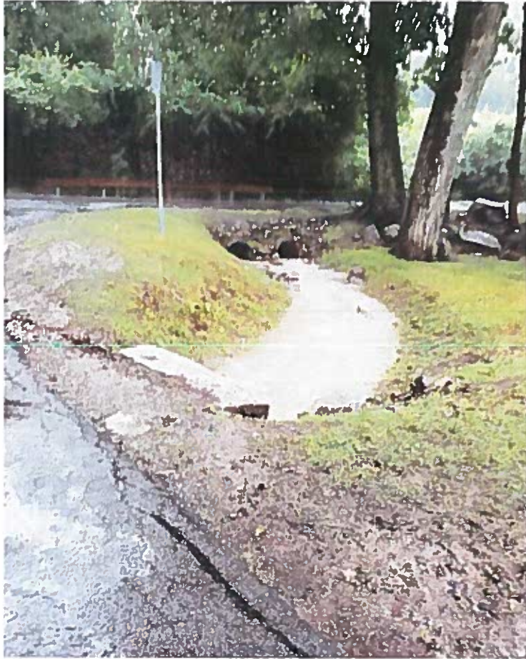
7/9/2021: Photo taken of the Howe Street Culverts at the driveway leading to the Water Treatment Plant.
