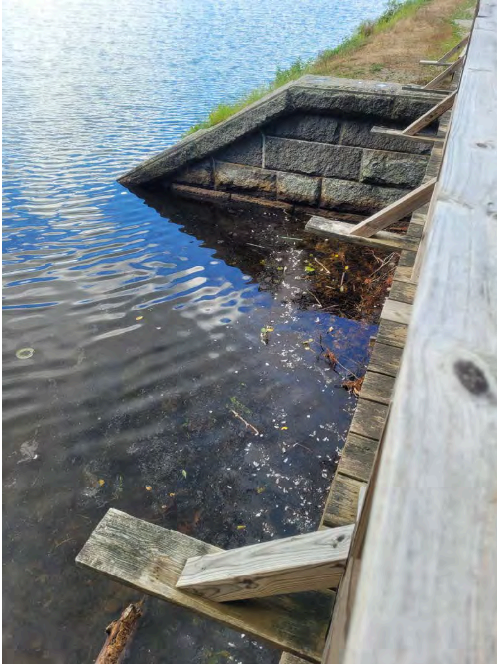
Photo 1 – View of reservoir side of pedestrian trail bridge. Standing on bridge viewing southwest.
