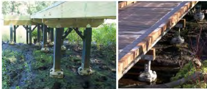
Photo #6: View of an example of a diamond pier wooden puncheon installed in a wetland.
