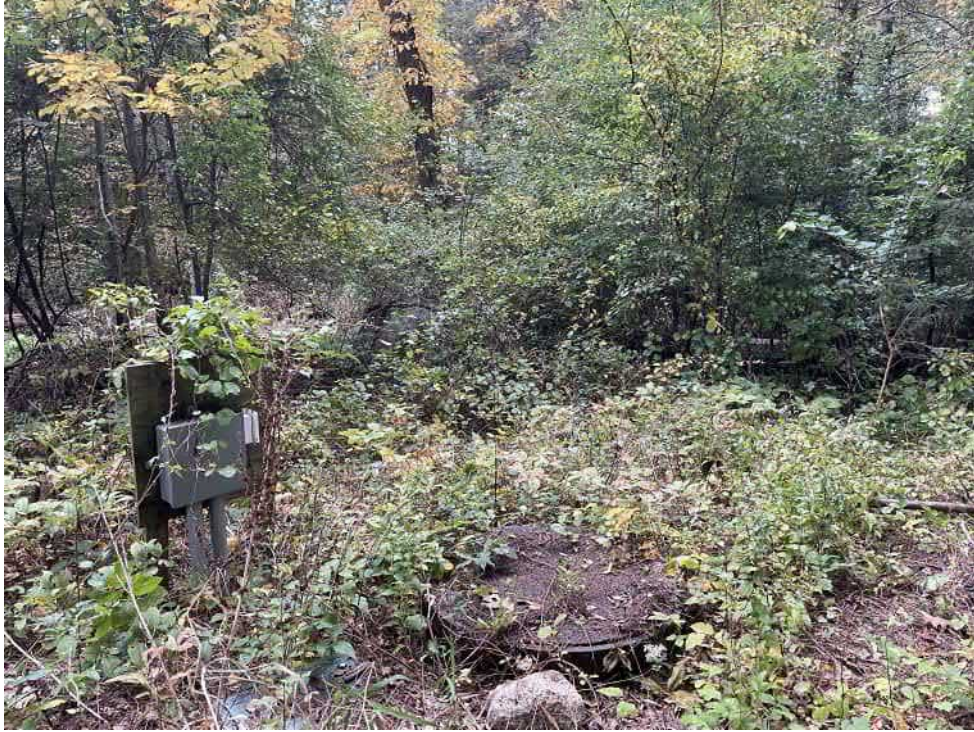
View of the Lower Pump Station—facing southwest.
