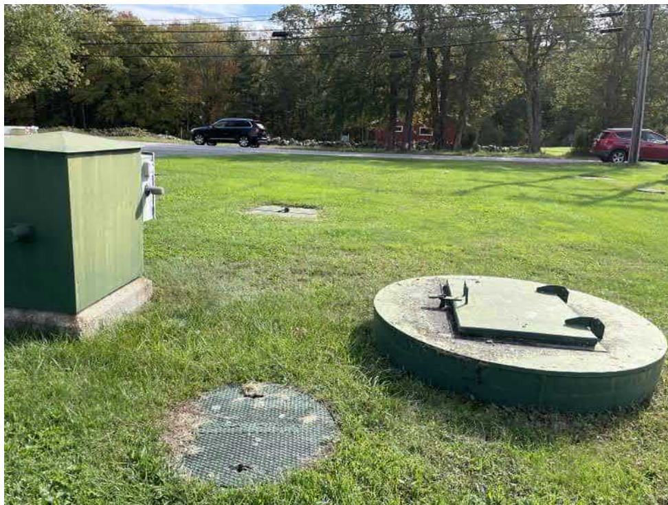
View of the Upper Pump Station—facing southeast.
