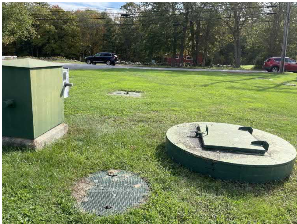
View of the Upper Pump Station—facing southeast.
