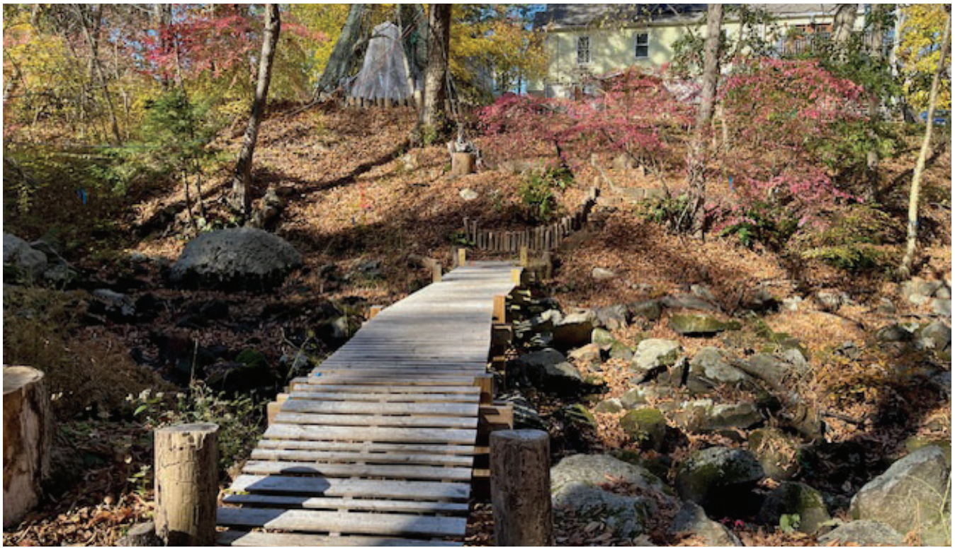
Photo #3: View of the wooden footbridge over the rocky stream. Note that posts sit on existing rocks.
