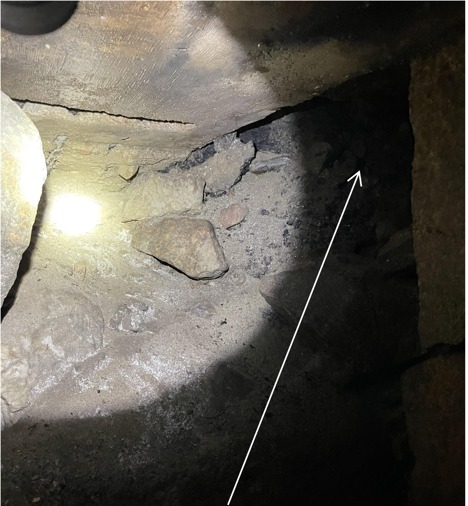
Cavity that has formed in the walls and bypassed the crown of the culvert.
