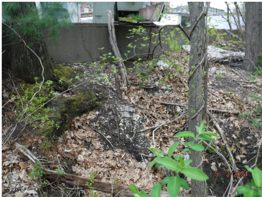
Photograph 10 : Existing pump house and drainage scour along retaining wall, facing west.
