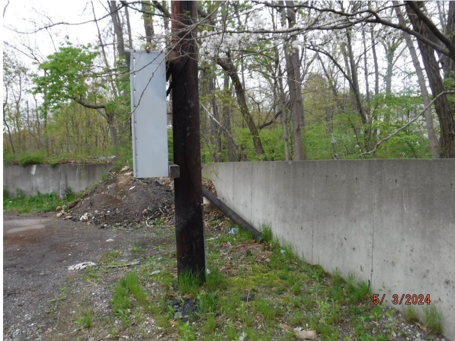
Photograph 19: View of existing utility connection to overhead wires along retaining wall, facing north.
