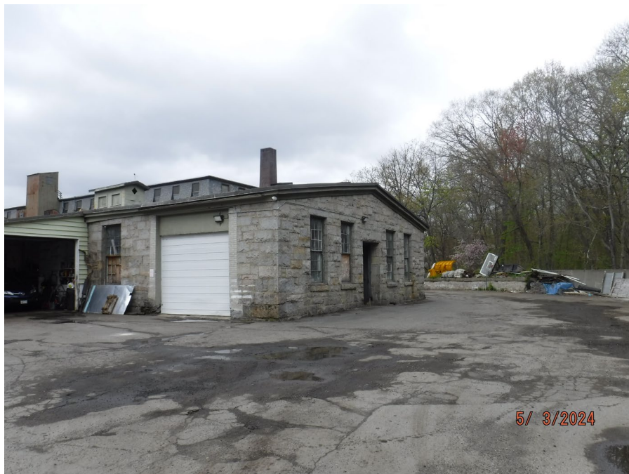
Photograph 14: Existing parking lot and degrading building within the Historic Mill Complex, facing north.
