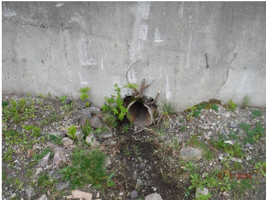
Photograph 18: View of existing deteriorating outlet pipe discharging into the Sudbury River, facing east.
