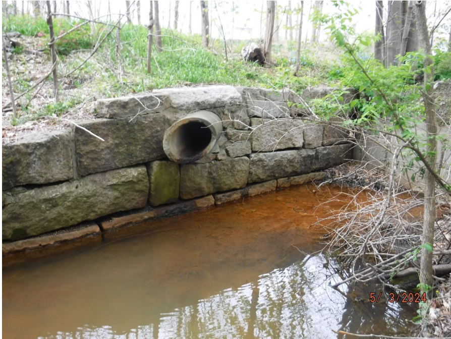
Photograph 1: View of existing concrete outlet structures along the southwestern corner of the property, within the canal off Main Street.
