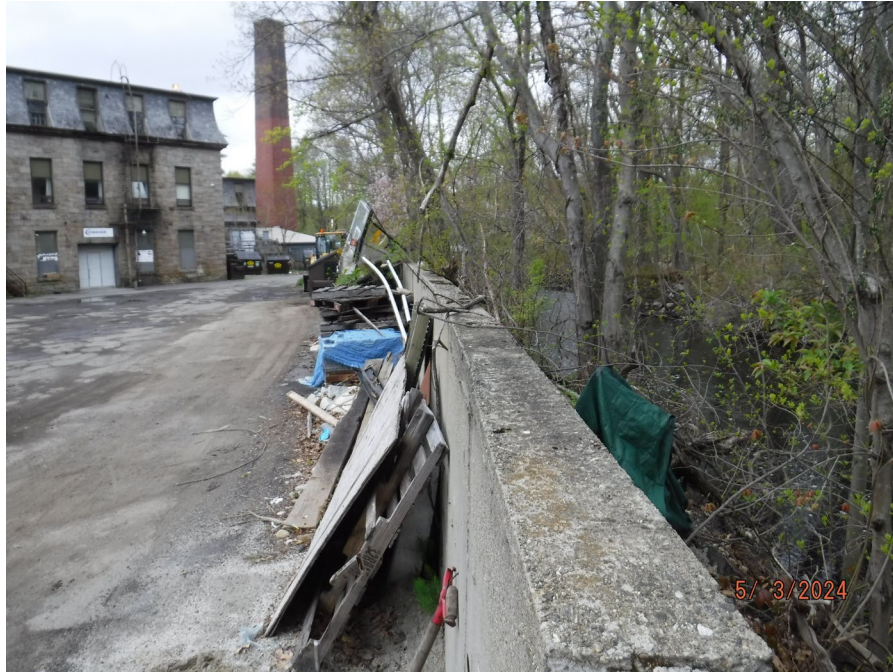
Photograph 15: Existing conditions of the retaining wall, degrading mill structure, and RFA, facing north.
