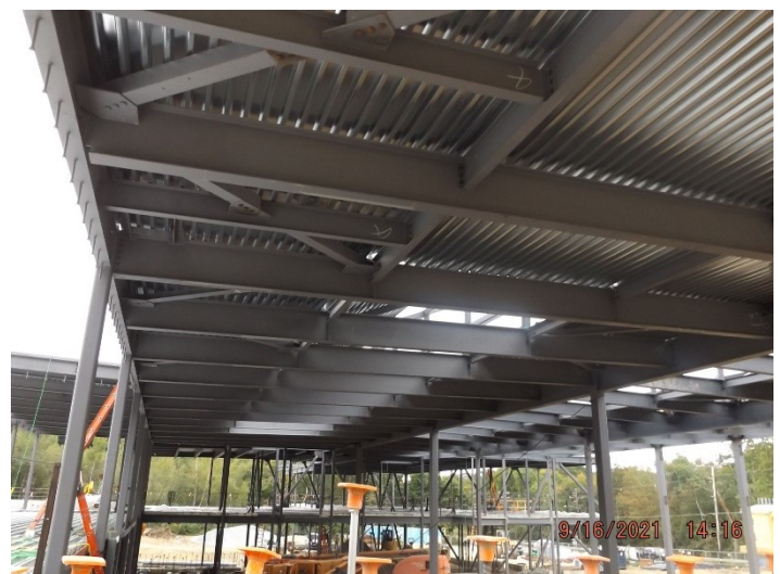
Photo depicts the progress of decking and detailing on the apparatus bay side.
