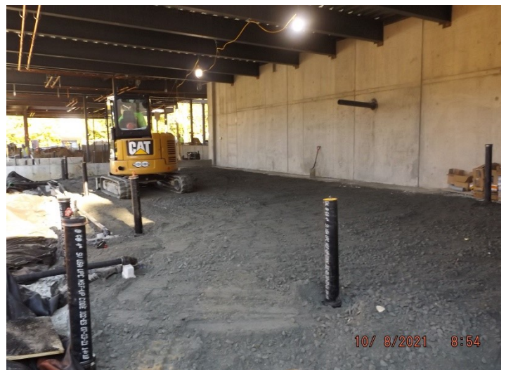
Photo depicts the progress of excavation and back filling of under slab utilities.
