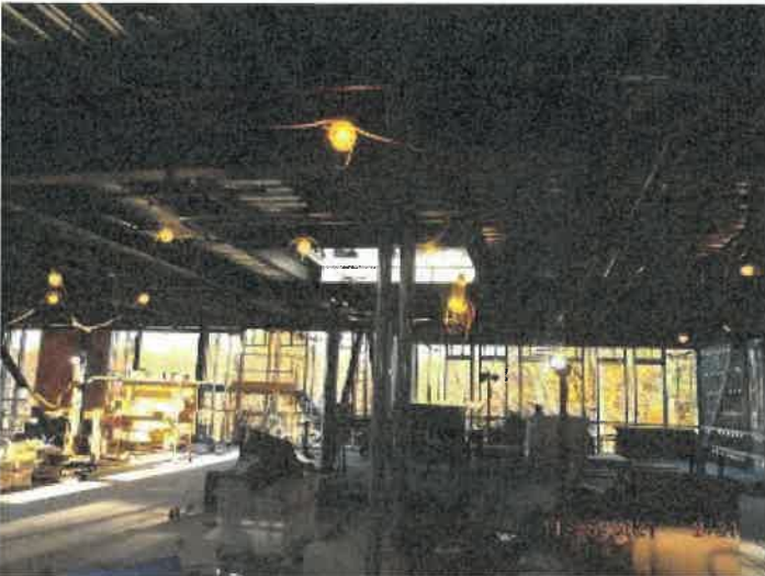
Photo depicts the progress rough electrical, fire protection and HVAC on second floor.
