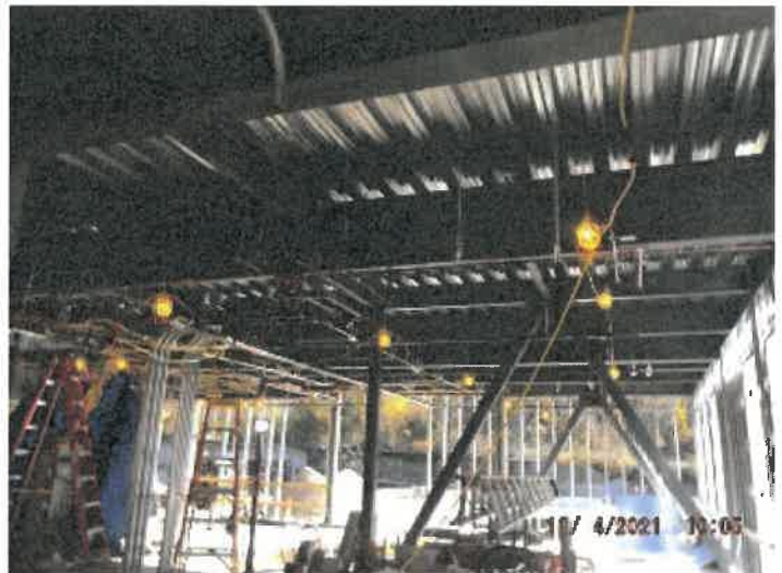
Photo depicts the progress rough electrical, fire protection and HVAC on the second floor
