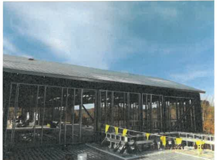
Photo depicts the progress of truss decking and framing of the third floor.
