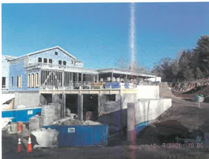
Photo depicts the progress of exterior sheathing, blocking and installation of CMU.
