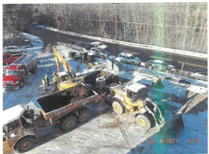
Photo depicts the progress of the front of the site along with underground utilities and drainage.
