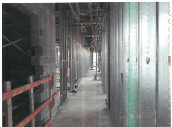
Photo depicts the progress of the third floor framing, sprinkler and HVAC
