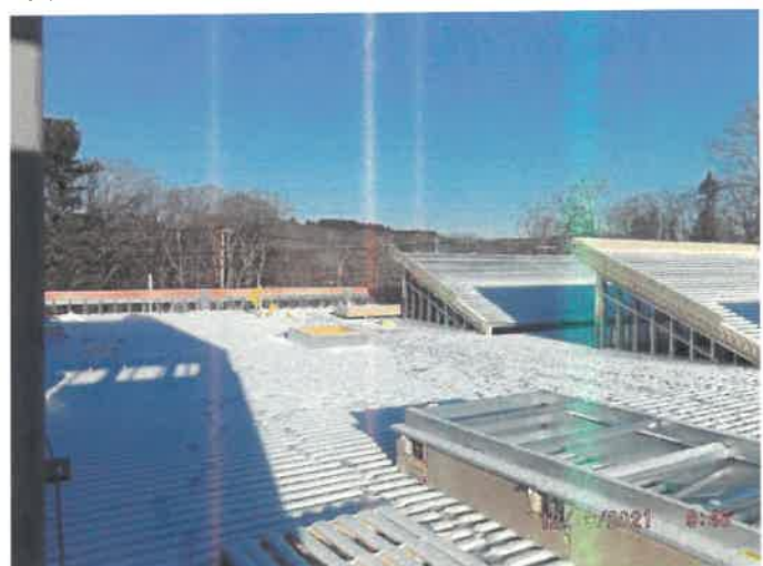
Photo depicts the progress of the apparatus bay roof framing and blocking.
