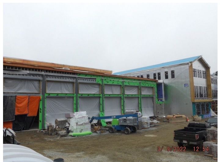
Photo depicts the progress of the parapet framing, sheathing, blocking, AVB, roofing and temporary enclosure to heat the building.
