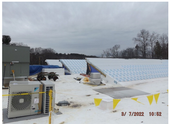
Photo depicts the progress of the apparatus bay roof, sawtooth roof framing and HVAC equipment.
