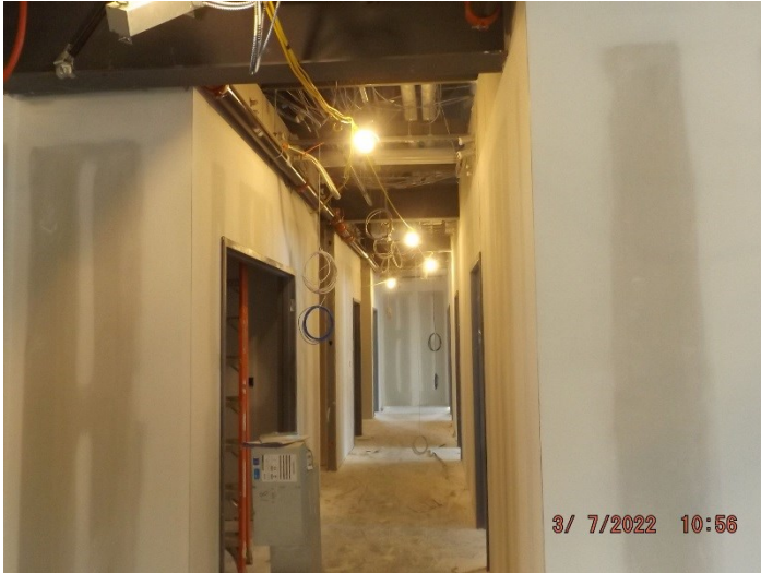
Photo depicts the progress of the third floor drywall, tape, mud, plumbing, HVAC, sprinkler system and electrical.
