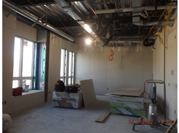
Photo depicts the progress of the Second drywall, HVAC, sprinkler system and electrical.
