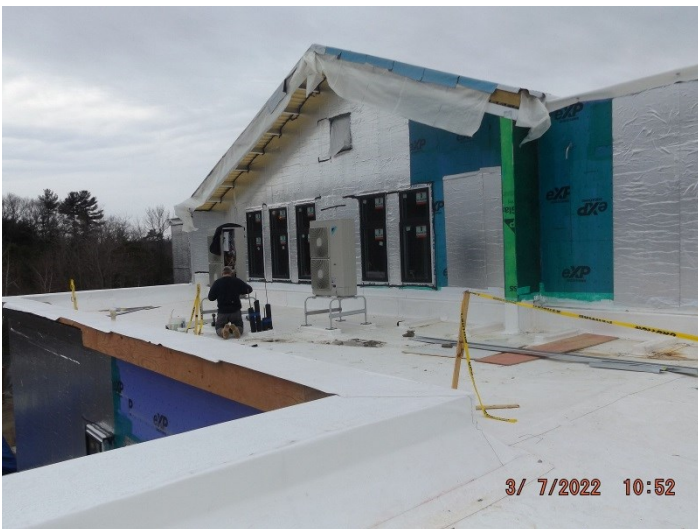
Photo depicts progress of the Apparatus bay roof, AVB, windows and HVAC equipment.
