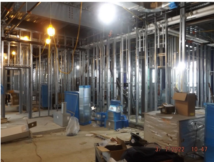
Photo depicts the progress of First floor framing, fire protection, plumbing, electrical and HVAC.
