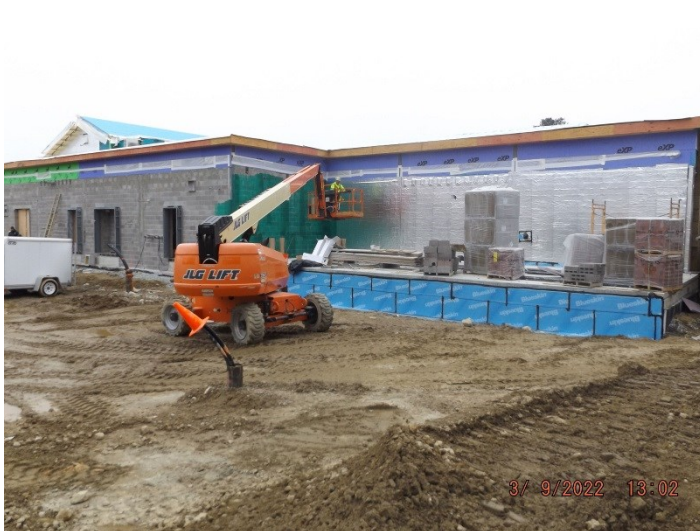
Photo depicts the progress of installation of door frames and AVB at rear of building.
