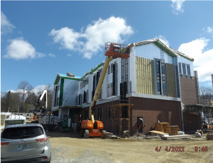
Photo depicts the progress of the AVB, window installation, window trim, brick, and secondary wall framing.
