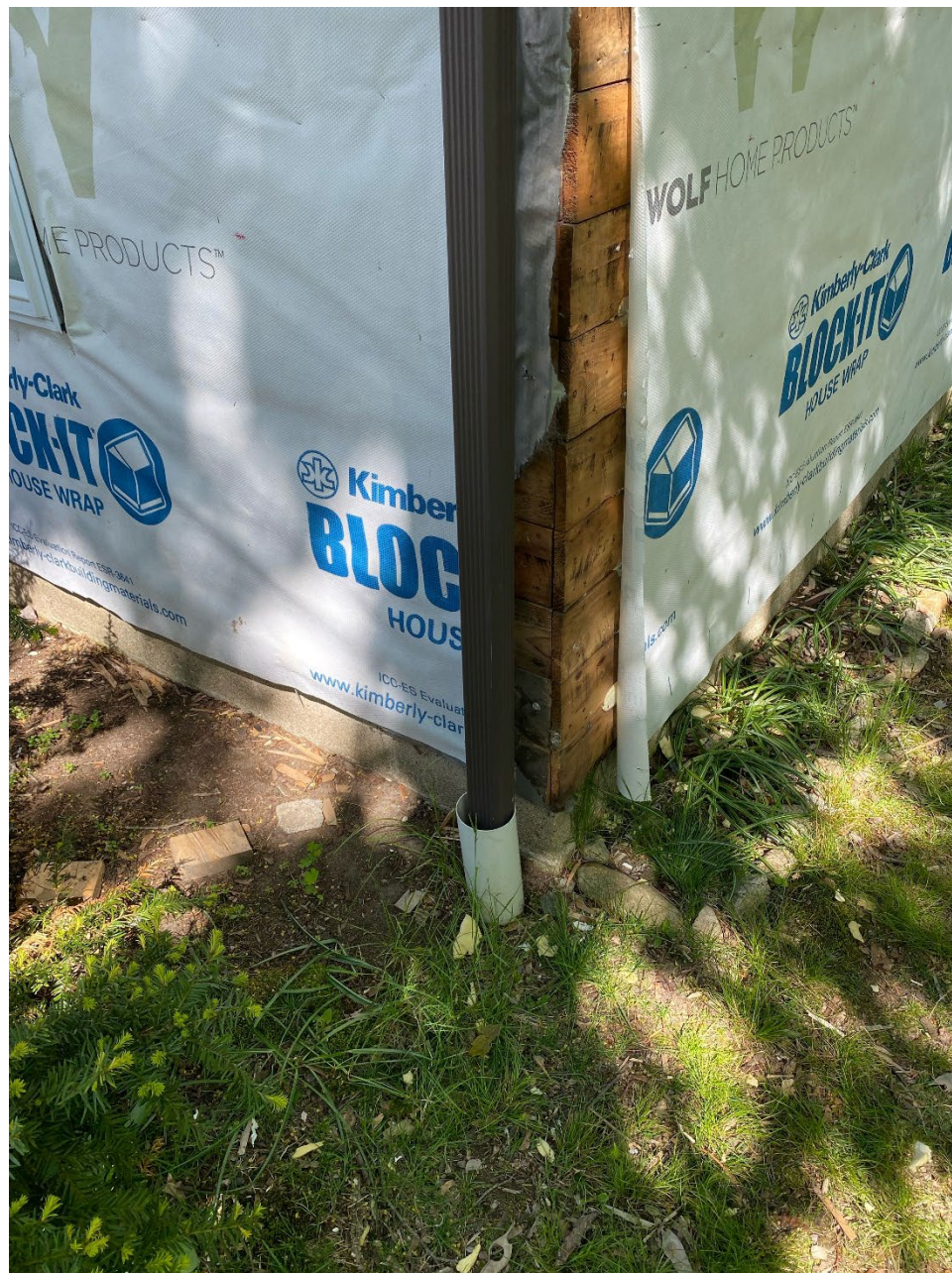
Photograph 2: View of PVC pipe and roof gutter located at the southwestern house corner, looking east.
