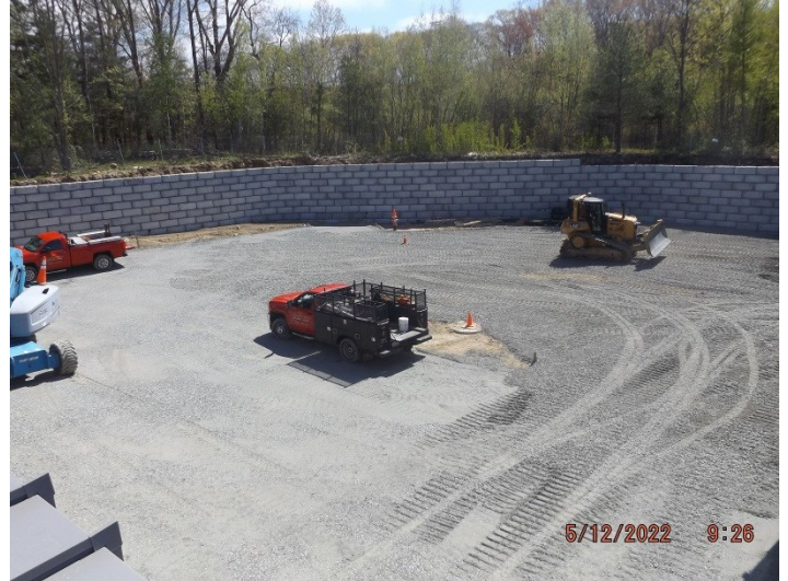
Photo depicts the progress of binder prep at the rear of site.
